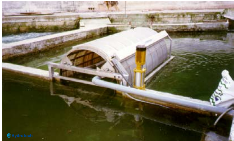
Drumfilter placed at the end of the race-way, ensures effective filtration conditions as particles are not disintegrated by piping or falling over weirs.
