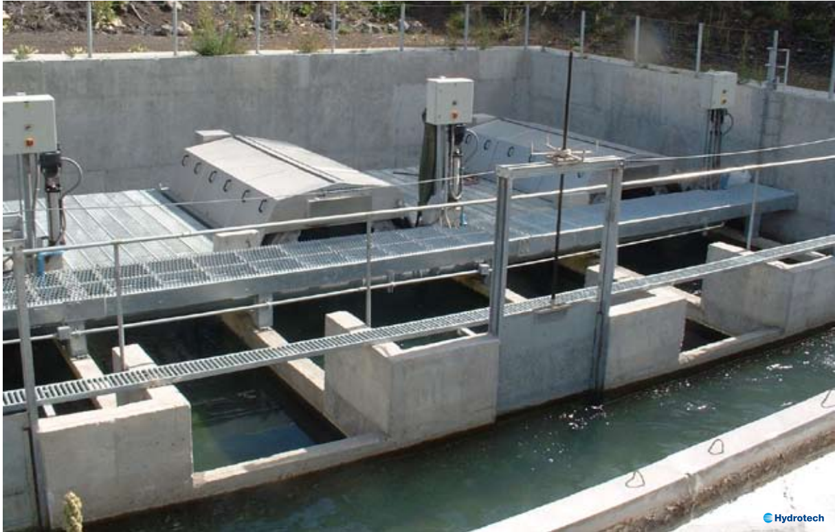
Outlet from a large salmon farm. Filters are installed in parallel, one common inlet- and outlet channel.
