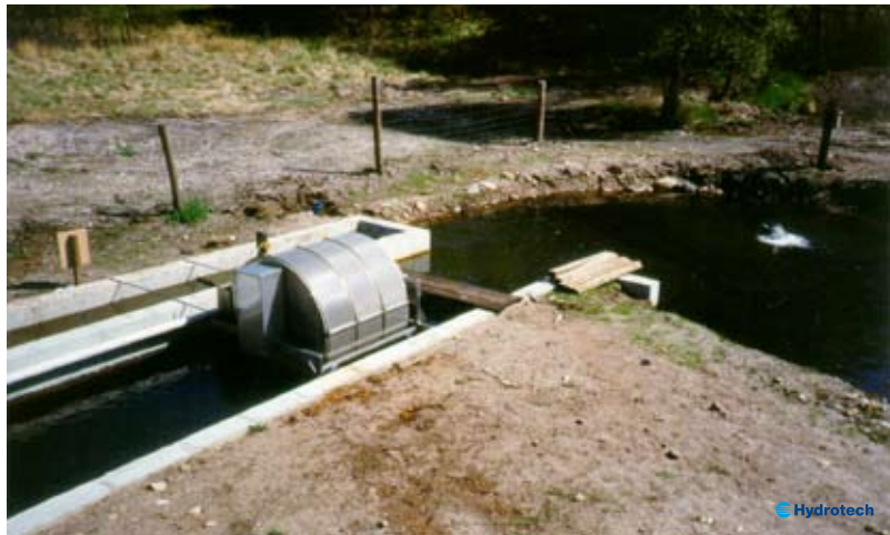
Drumfilter placed at the end of an earth pond. After the filter is space for biofilter for conversion of ammonia and further reduction of organic material.
